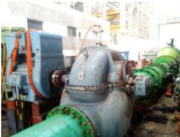
Pump testing arrangement
