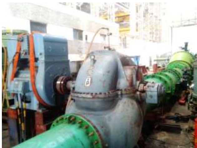
Pump testing arrangement
